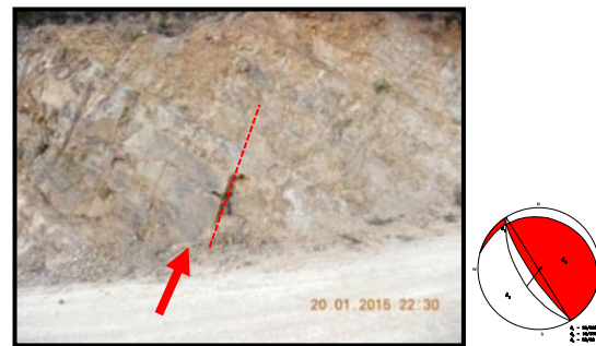
Figure (15). NNW-SSE trending reverse fault on the sandstone and siltstone unit of the Loi-an Group (20° 24' 58.7" N, 96° 38' 28.1" E) Photo Facing - SE
