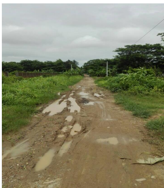
Figure (16) Poor road in rural area of Hinthada Township. (Source: Field Observation)
